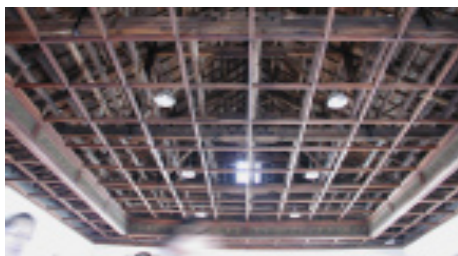
將室・原有天花板拆除，露出洋式屋架。 Western roof truss exposed when the ceiling was dismantled.
